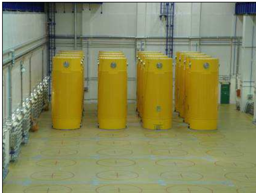
Fig. 4.4 Storage hall in SFSF Temelín
