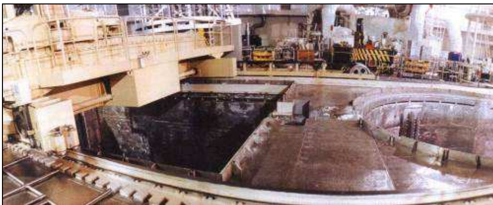
Fig. 4.3 Uncovered SF pool at NPP Temelín
