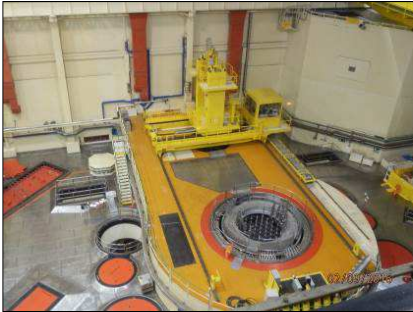
Fig. 4.1 SF pool and transfer cask shaft during reactor refueling
