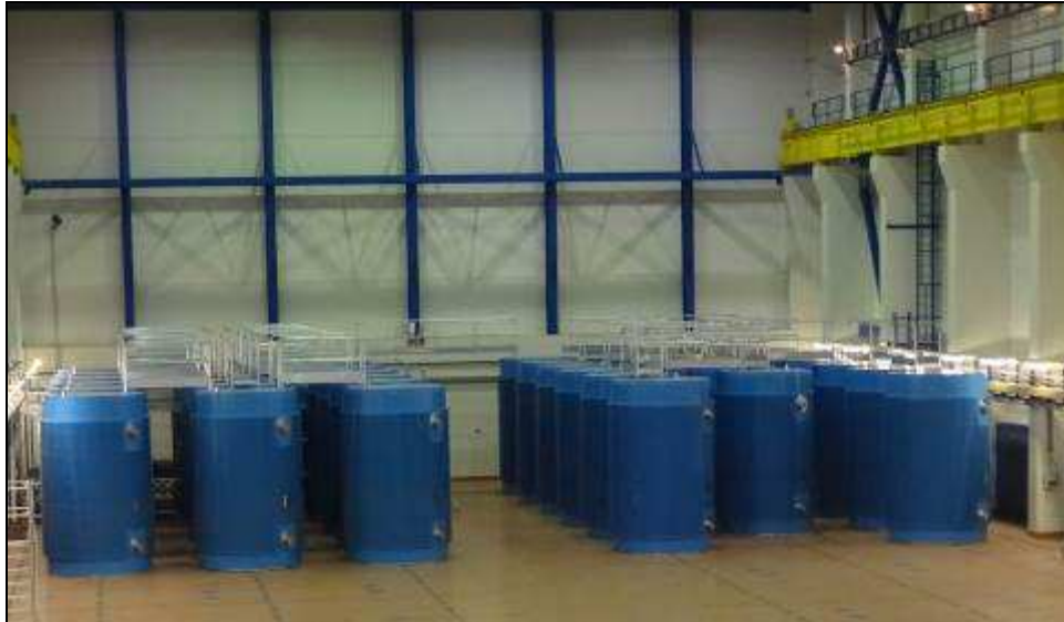
Fig. 4.2 Storage hall in SFSF Dukovany
