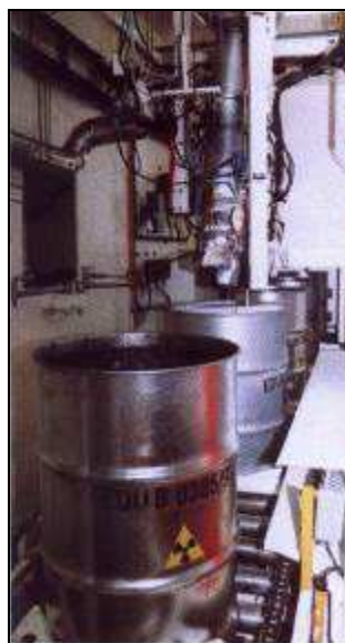
Fig. 4.5 View of a bituminization line to process liquid RAW
