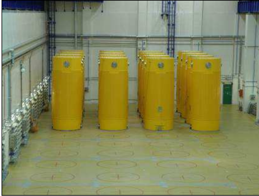
Fig. 4.4 Storage hall in SFSF Temelín
