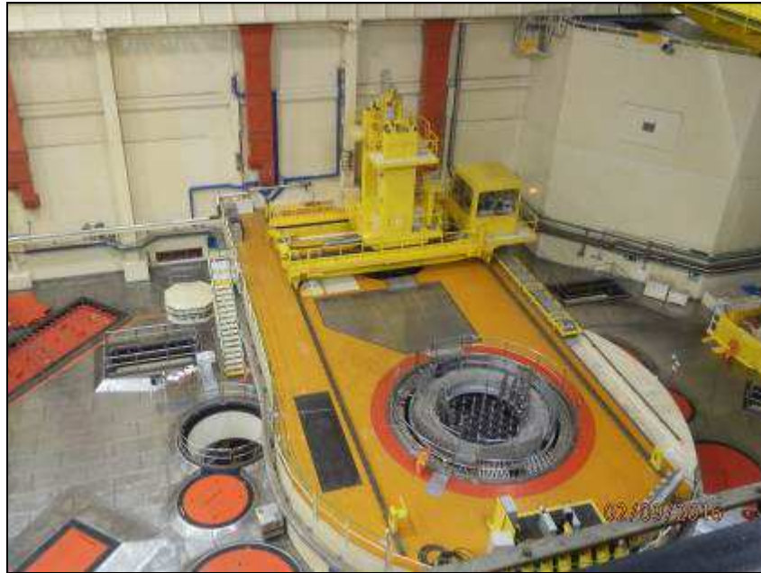
Fig. 4.1 SF pool and transfer cask shaft during reactor refuelling
